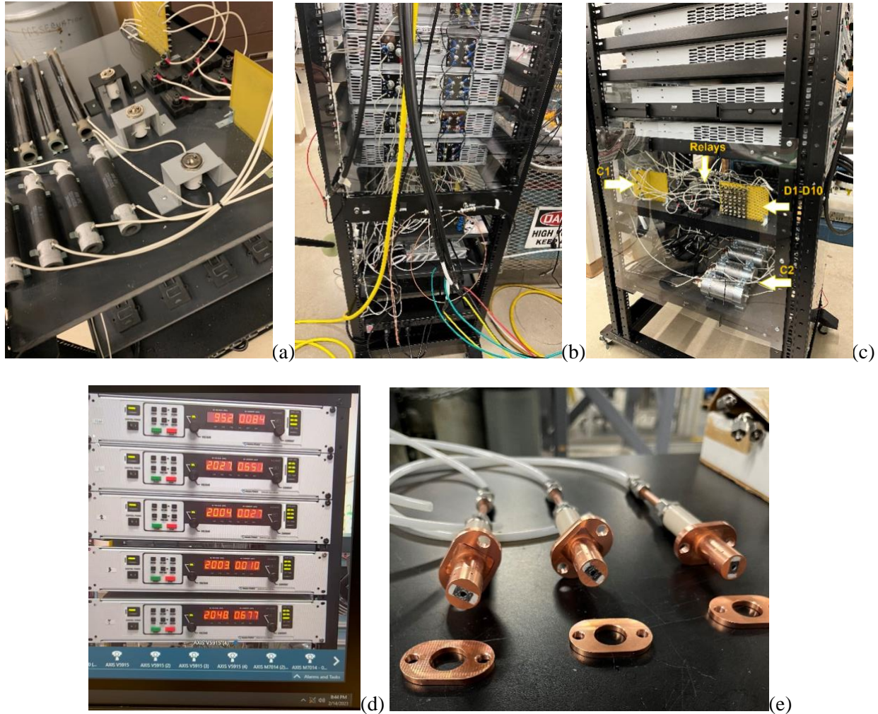
Figure 3. Major components and failure testing result: (a) - Close up of PS components during initial assembly and wiring (b) – back side of the PS at wiring; (c) – side view of the PS with major components; (d) - failure test, all boxes in operation, #1, #2 and #4 are loaded; (e) – three PIMs before wind tunnel installation.
